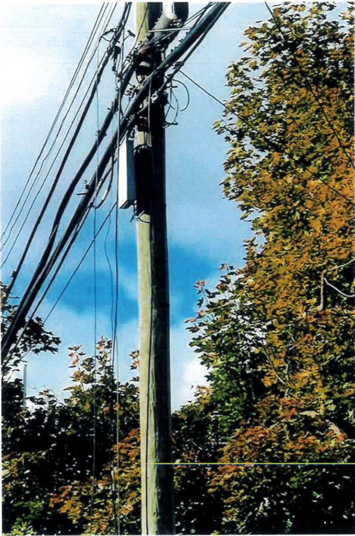
Utility pole on property with many wires hanging down - since corrected
