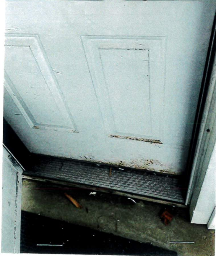
Rusted rear door
