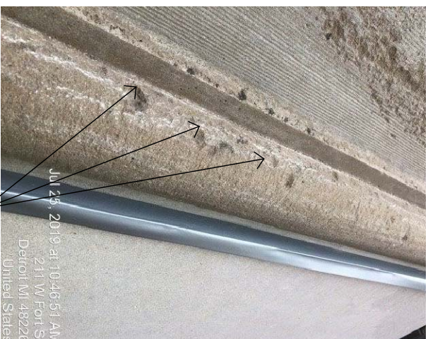
Damaged Locations At Existing Building Base
