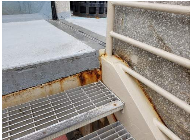
Section loss at stair/bridge connection
