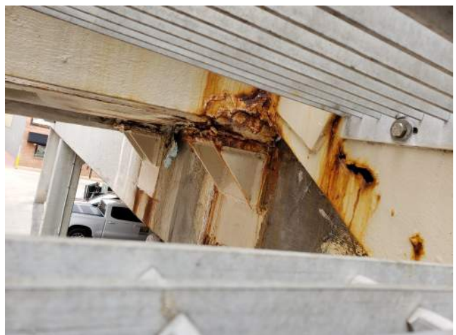
Section Loss at bridge/parking structure connection
