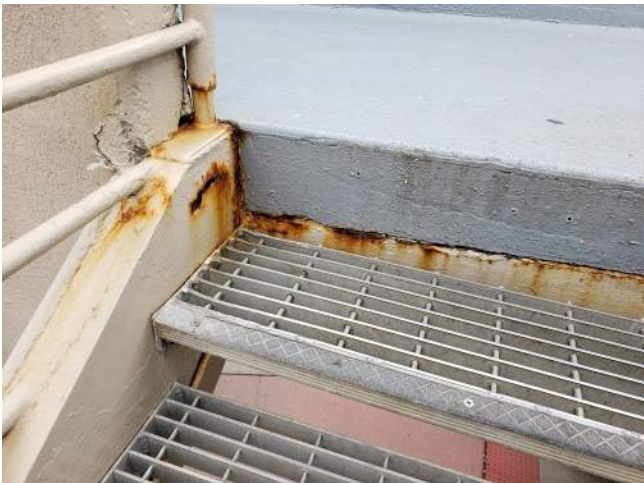
Section loss and holes at stair stringer
