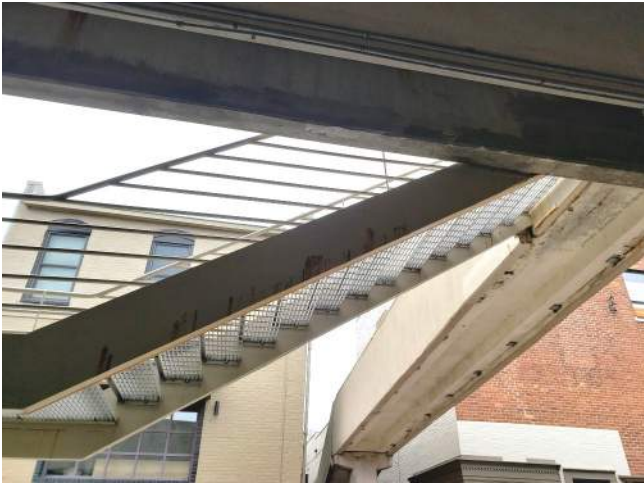
Section loss along interior stringer
