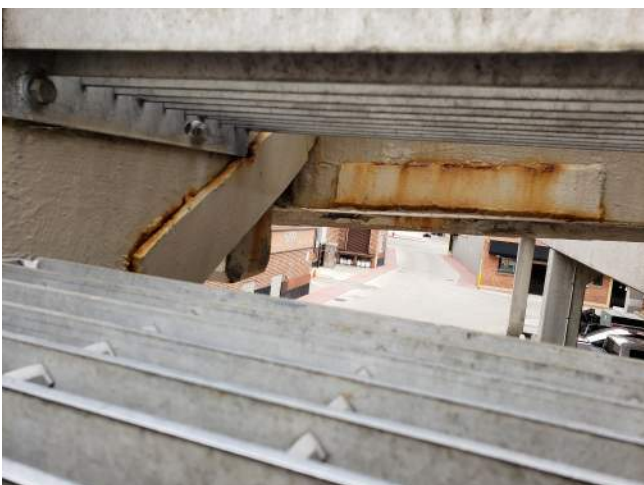
Previous steel repairs at stairs
