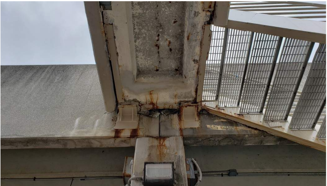
Concrete delaminations and corrosion of precast connections at spandrel wall
